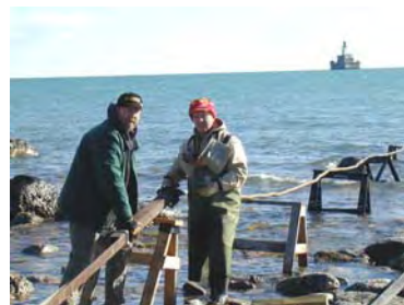
Lions Ken Walker (left) and Norm Muench installing a protective tube around the power line to the lighthouse where it enters Lake Huron at DeTour Point.
