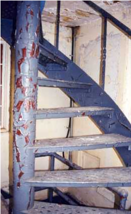
Steps of DeTour Reef Light prior to restoration
