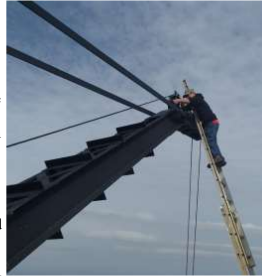
Terry Breiler applying grease to the cables on top of the crane
