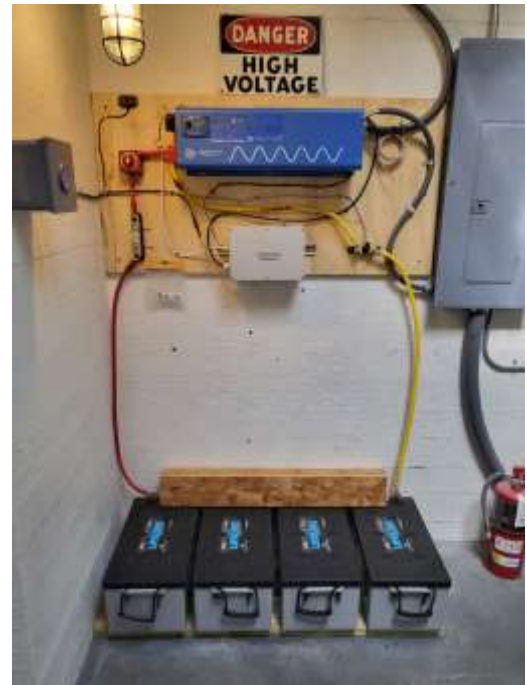
Batteries, inverter, generator control box
