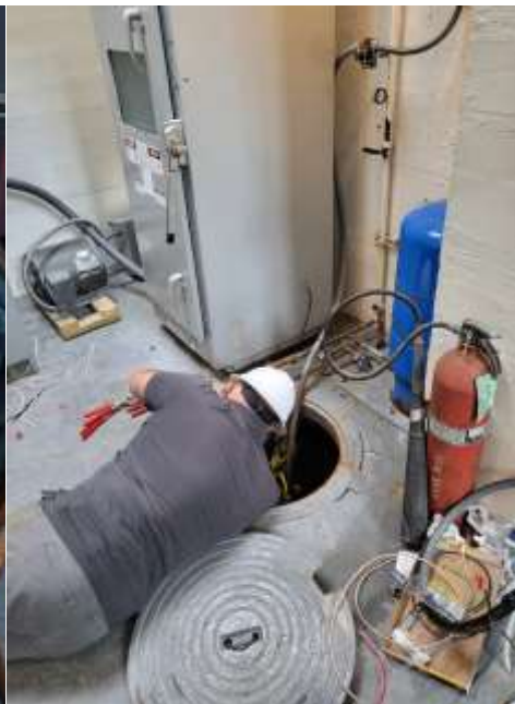
Brent working on a leaking well pump.
